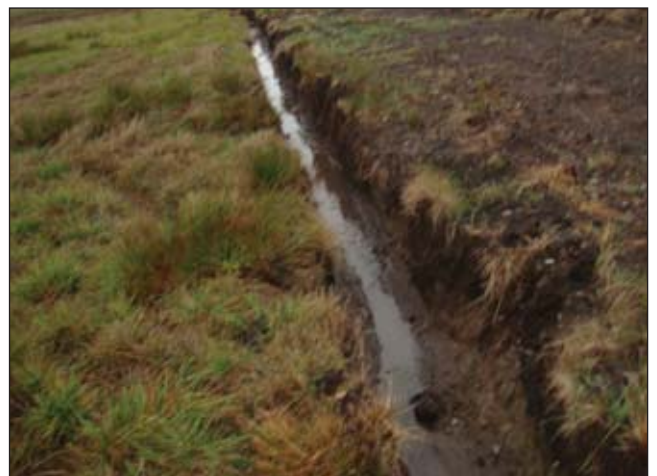
PHOTO 10: View southward of manmade drainage ditch (DCH 1) that flows south to north through the eastern portion of the study area.
